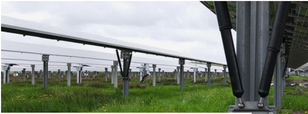
Figuur 2: single-axis tracking systeem, Le Pouzin II, France
